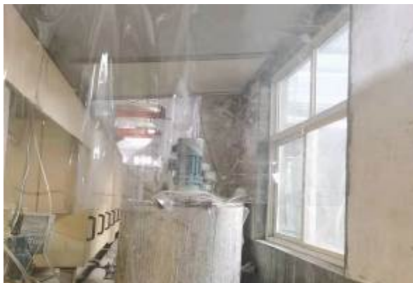
调胶废气收集软帘
